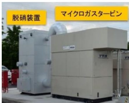
50kW (100% NH 3 ) Micro Gas Turbine
