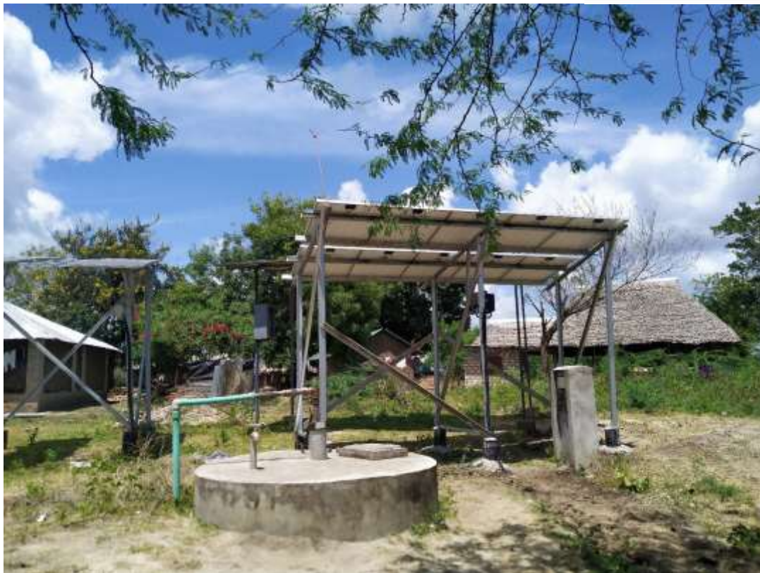
Solarized boreholes at Moa that serves approximately 3,500H/H, in Lamu County.
